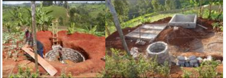
Left: Biogas system under construction in January. Right: It is now almost ready to produce gas for cooking. The gas pipe will be con-
